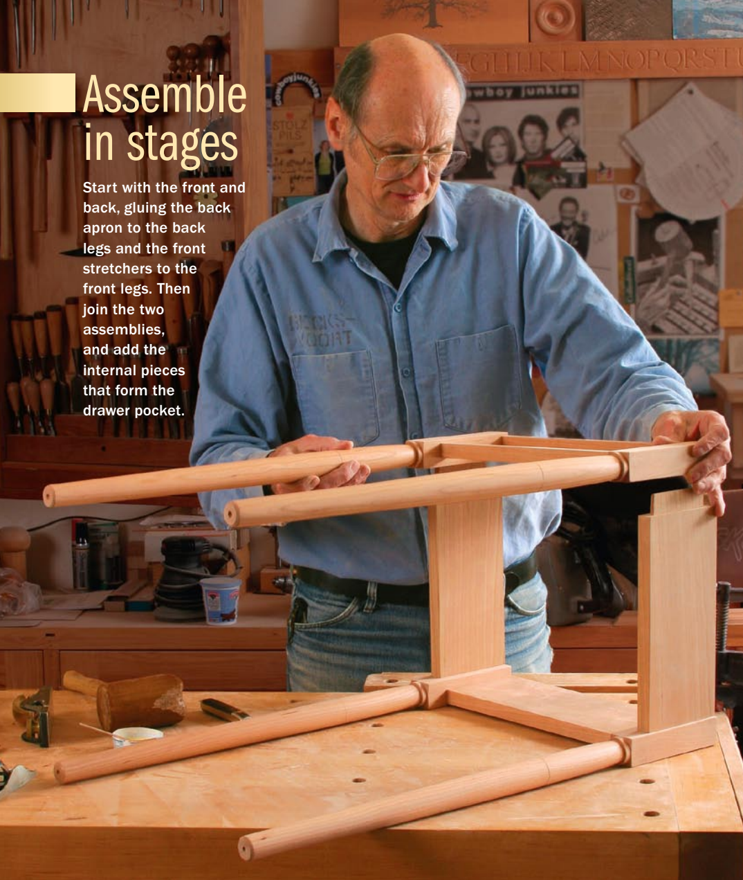
Complete the base. After the front and back of the base are dry, add the side aprons.
